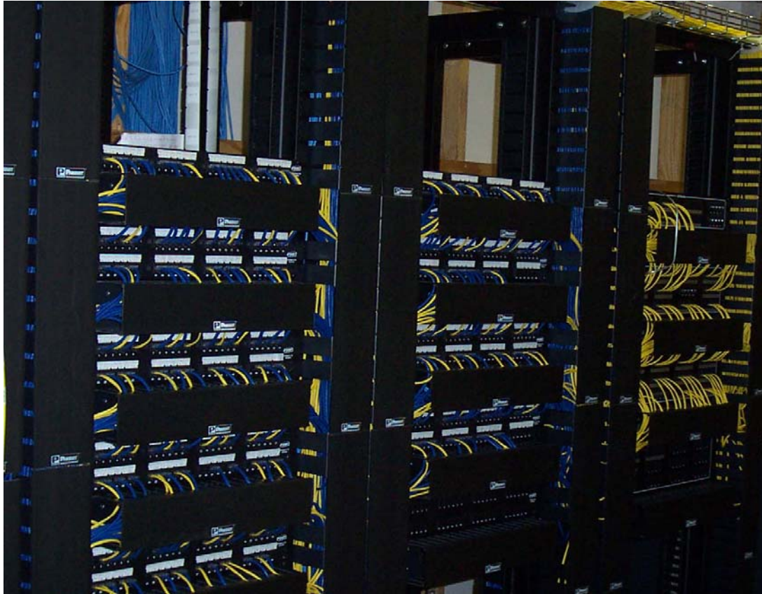
Cable Management picture 1
